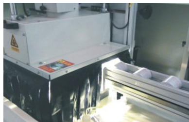
UV Curing System
